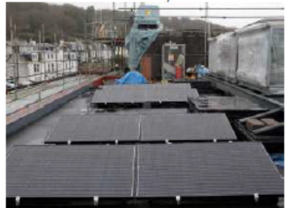
Main Roof – The Solar PV panels insitu adjacent West Elevation.
