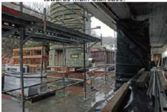
General View: Auditorium West wing (looking North). NB: base of site crane visible.
