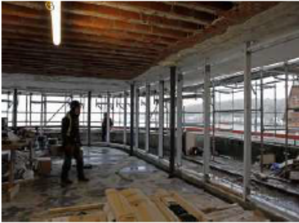
New curtain walling line to the new Exhibition/Function room (towards Argyll St)
